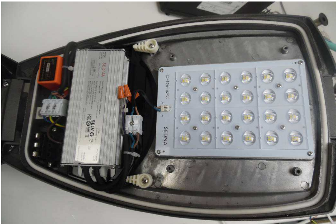
Inside the EUT (post IPX6 test)
