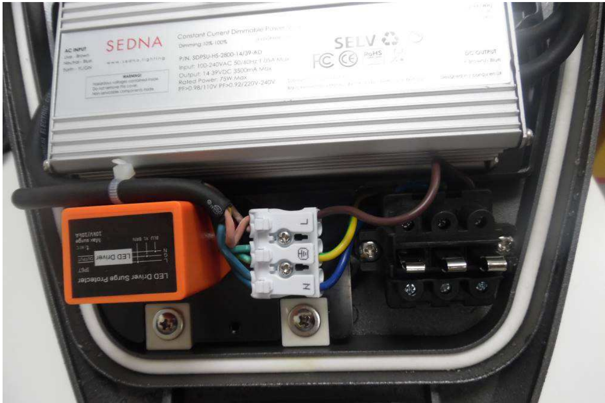
Inside the EUT (post IPX6 test)
